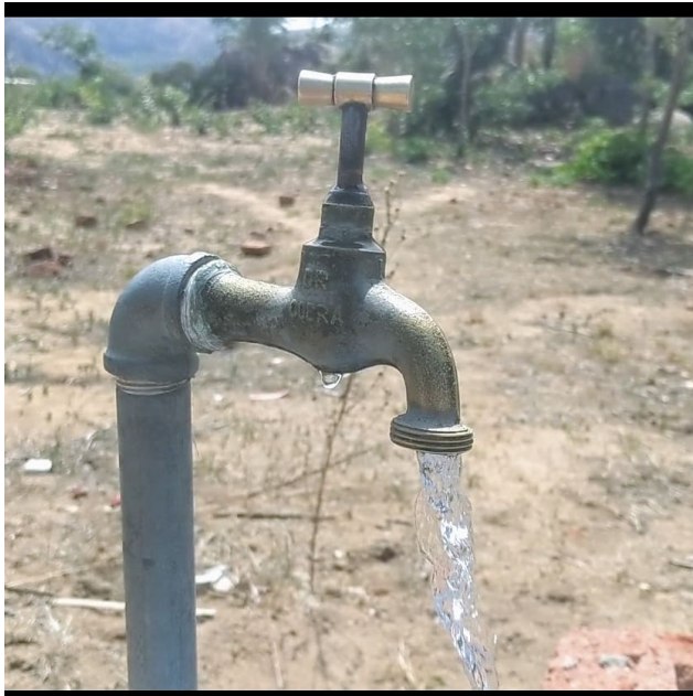
Figure 2: Clean tap water to drink
